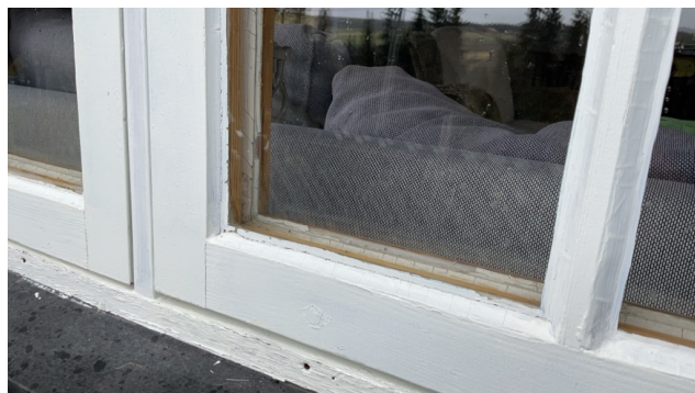
Sprekkdannelse i kitt
