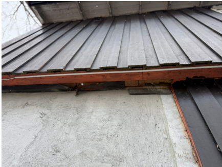
Manglende tetting under bjelkelag.
