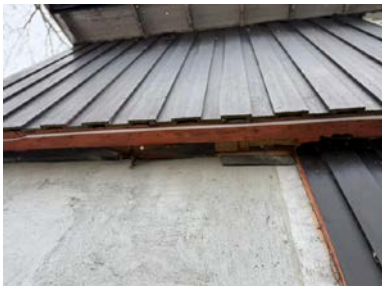
Manglende tetting under bjelkelag.
