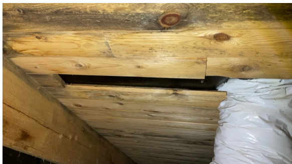
Noe manglende undertak.
