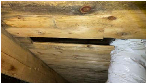
Noe manglende undertak.
