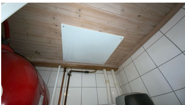
Fordelerskap i himling.
