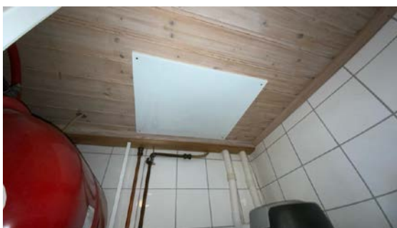
Fordelerskap i himling.
