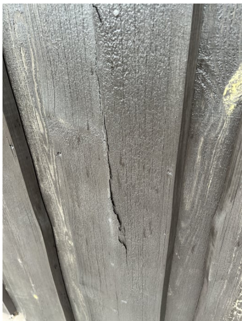
Sprekker i panel.
