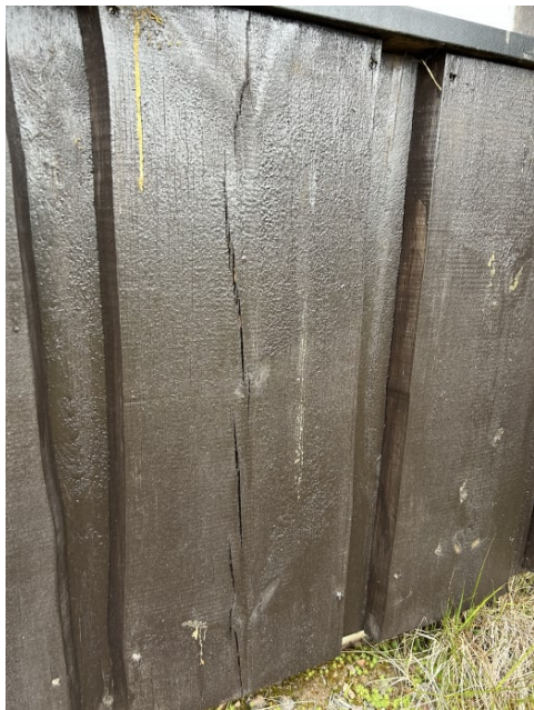
Sprekker i panel.
