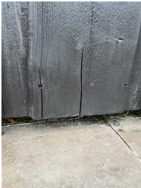
Sprekker i panel.
