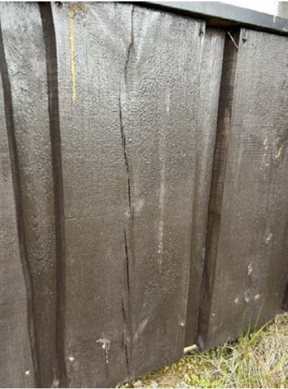
Sprekker i panel.
