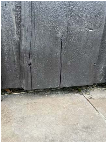
Sprekker i panel.
