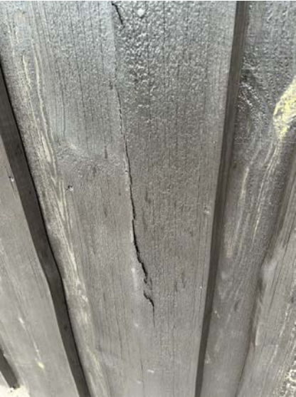
Sprekker i panel.
