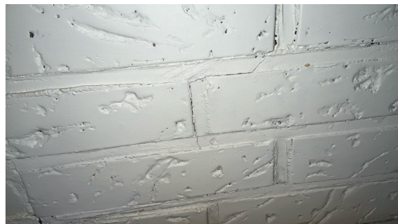
Riss i pipe/brannmur st
