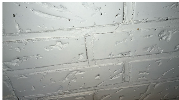
Riss i pipe/brannmur st
