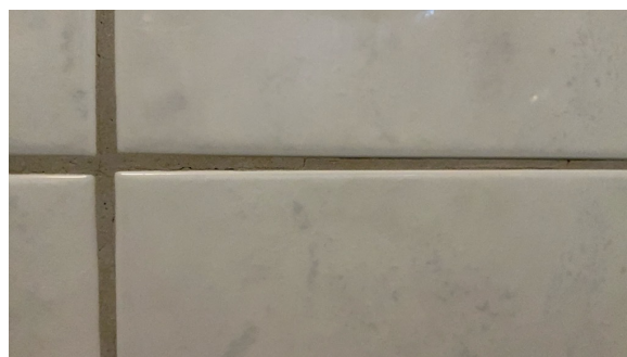
Riss i flisfuge
