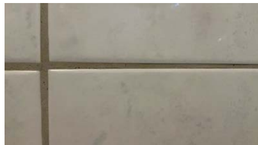
Riss i flisfuge
