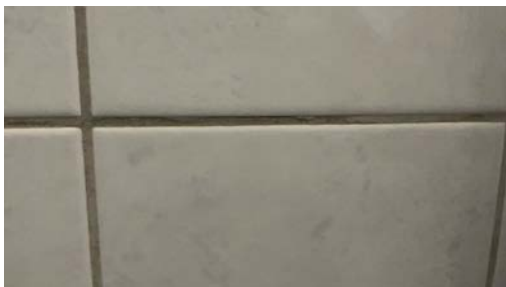
Riss i flisfuge
