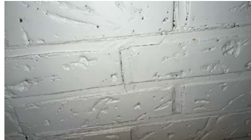
Riss i pipe/brannmur st
