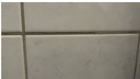
Riss i flisfuge
