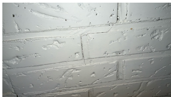
Riss i pipe/brannmur st
