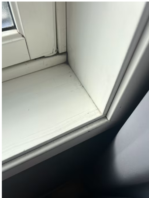
Fuktskade i foring.
