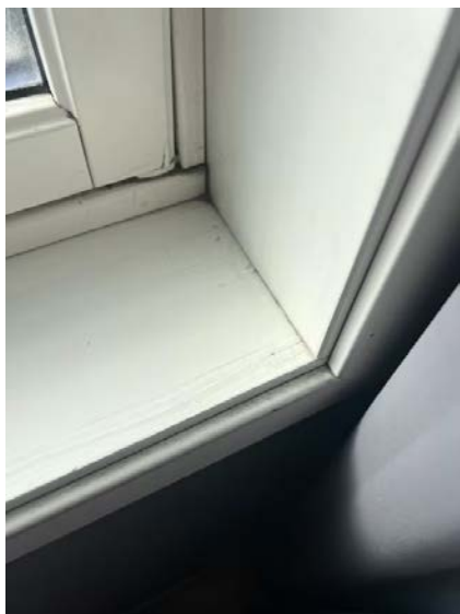
Fuktskade i foring.
