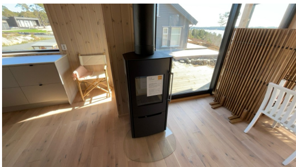
Montert oven i stue.
