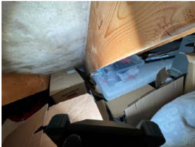
Mye merker i undertaket, skyldes fuktig inneluft.
