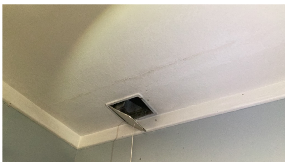
Slitasje i himling.
