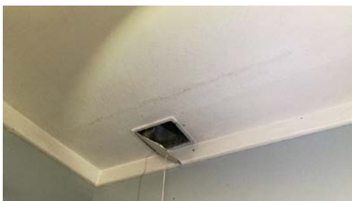
Slitasje i himling.
