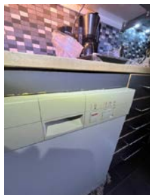
Fuktsvelling over oppvaskmaskin
