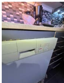
Fuktsvelling over oppvaskmaskin
