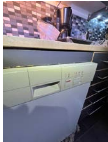
Fuktsvelling over oppvaskmaskin
