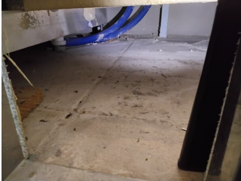
Røropplegg under badekar
