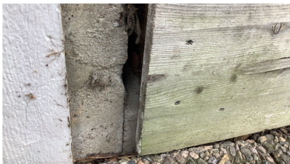
Mangelfull trelem foran luke.
