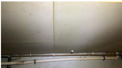
Svellskader i himling.
