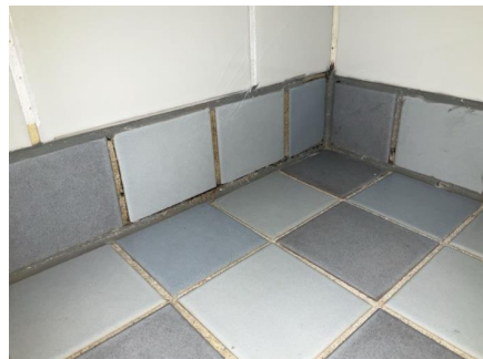
Sprekker i flisfuger. Misfarginger i flisfuger.
