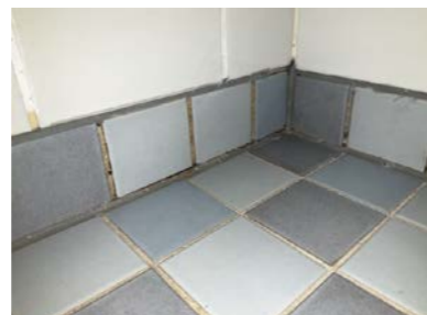
Sprekker i flisfuger. Misfarginger i flisfuger.
