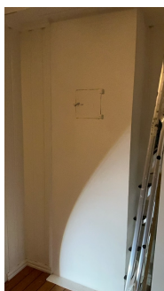
Mangler plate under sotluke/feieluke
