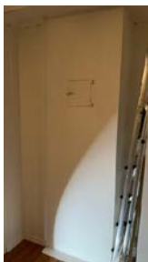
Mangler plate under sotluke/feieluke
