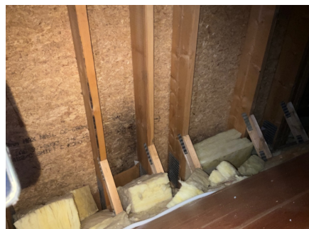
Mørke flekker i undertaket.
