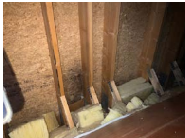
Mørke flekker i undertaket.
