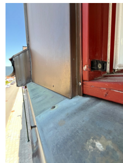
Sprekker i karm, noe malingsslitt
