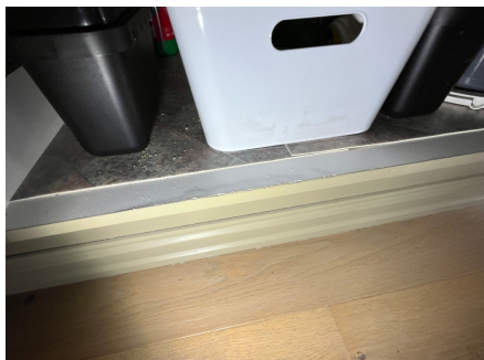
Fuktsvelling i bunnplate
