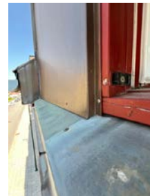
Sprekker i karm, noe malingsslitt
