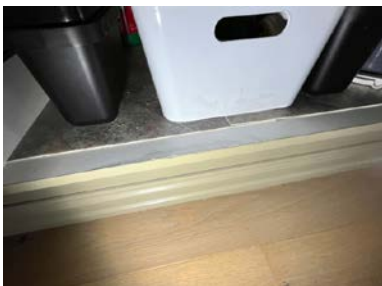
Fuktsvelling i bunnplate
