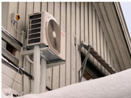
Ising under varmepumpe
