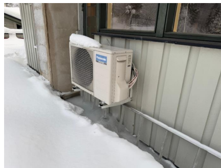
Ising under varmepumpe
