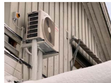
Ising under varmepumpe
