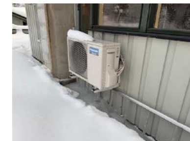
Ising under varmepumpe
