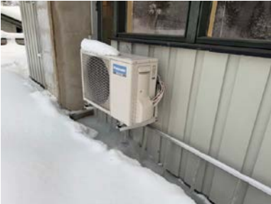
Ising under varmepumpe
