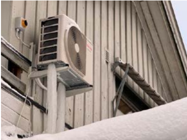
Ising under varmepumpe
