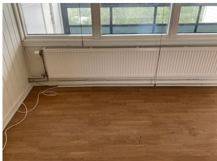
Radiator i stue, tilkoblet sentral oppvarming.
