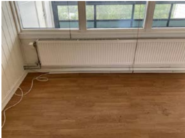
Radiator i stue, tilkoblet sentral oppvarming.
