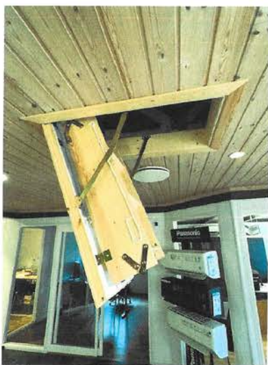
Feilmontert lofts luke.
