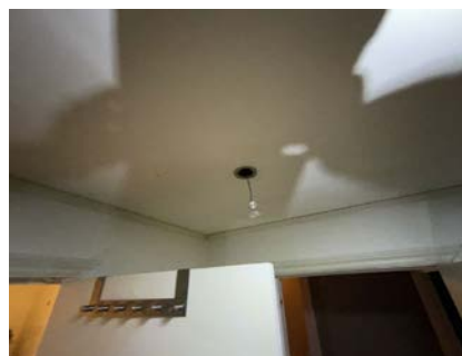
Downlight i gang.
