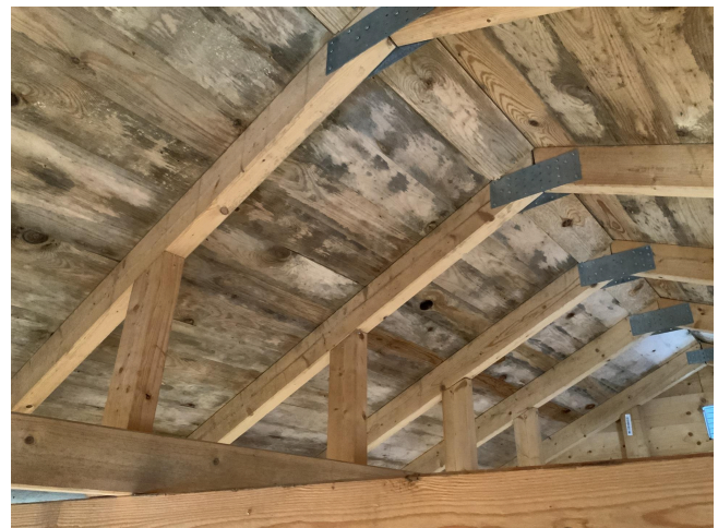
Fuktmerker i undertaket.
