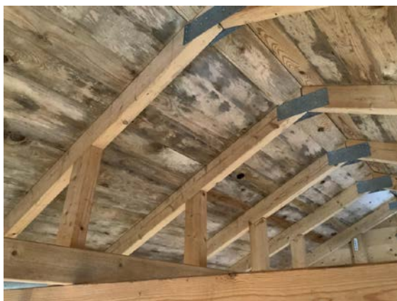
Fuktmerker i undertaket.
