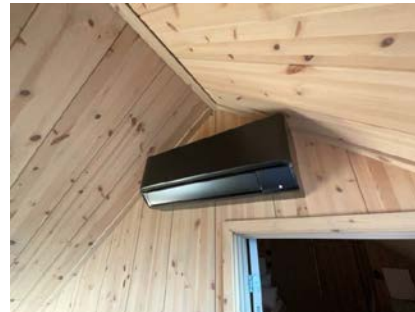
Varmepumpe, innvendig aggregat.
