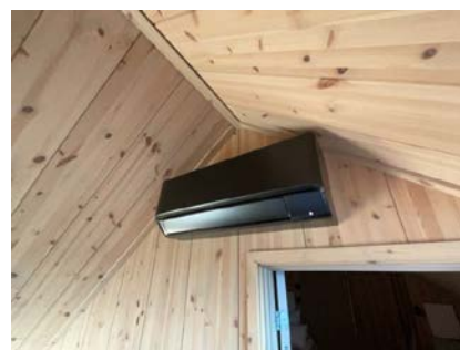
Varmepumpe, innvendig aggregat.
