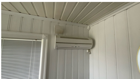
Varmepumpe, innvendig aggregat.
