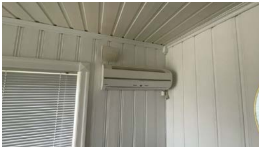
Varmepumpe, innvendig aggregat.
