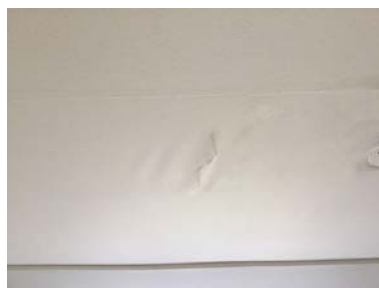
Fuktskjolder i himling.
