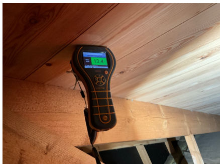
Normale fuktverdier i undertaket.
