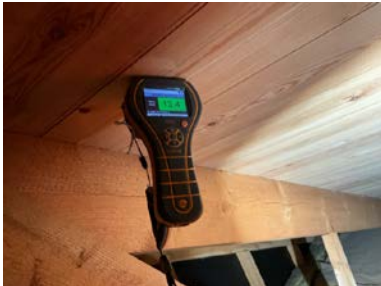
Normale fuktverdier i undertaket.
