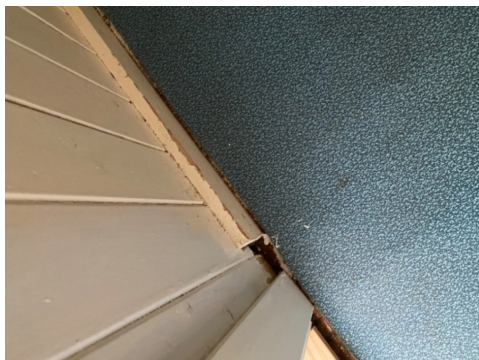
Manglende listverk, (bod)
